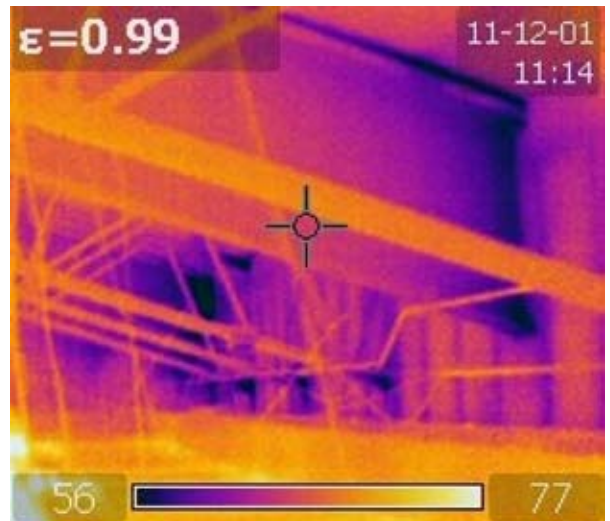
Figure 1: Infrared scan of structural steel balcony beam cantilevering out from a structure.
